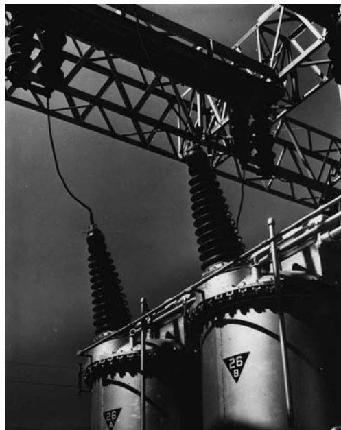
photo © Franklin D. Roosevelt Presidential Library ■ TVA Transmission Line, completed in 1936. This tall tower is a part of the Tennessee Valley Authority (TVA) high tension transmission line linking Norris Dam with Wilson Dam at Muscle Shoal, AL.
